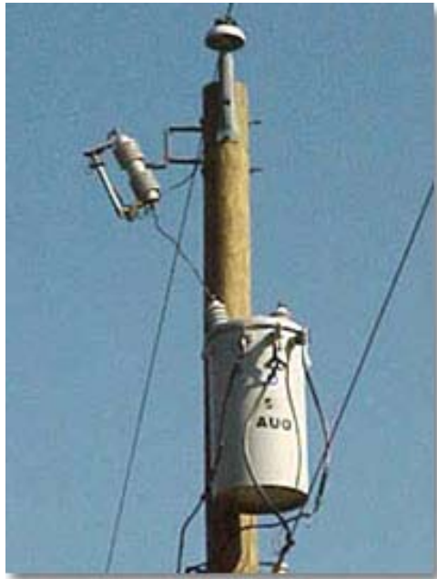
Figure 2: Typical Pole-mounted Transformer
